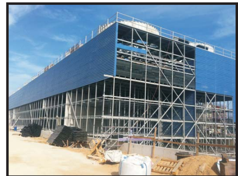
Cooling Tower Application
